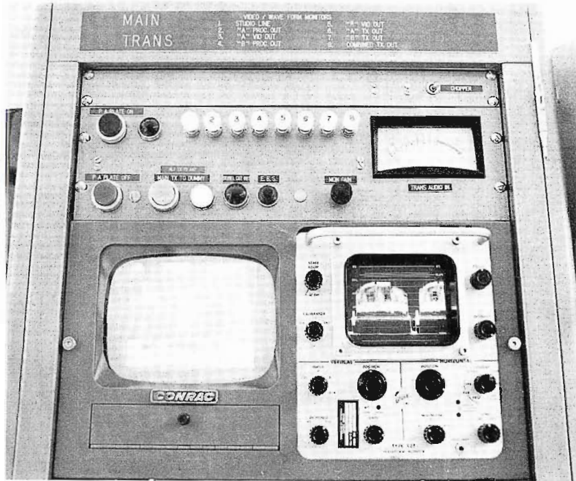
Close-up of left console control panel showing controls for monitoring output and for accomplishing transmitter changeover.
