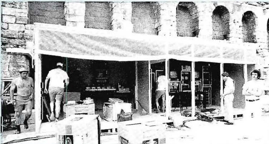
A "house"—complete with air conditioning—was constructed in the Ampitheatre for the Control Room gear.
